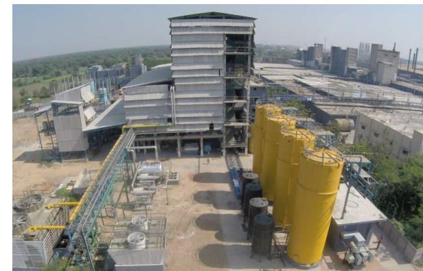
Multiple Effect Evaporator Plant (MEEP)
