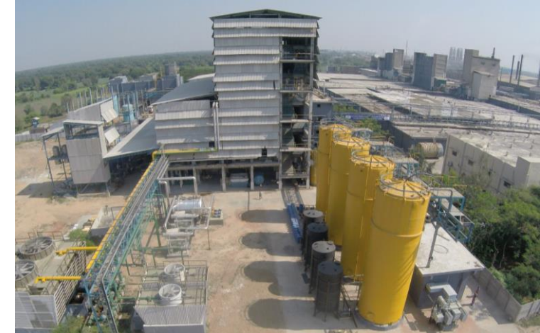
Multiple Effect Evaporator Plant (MEEP)
